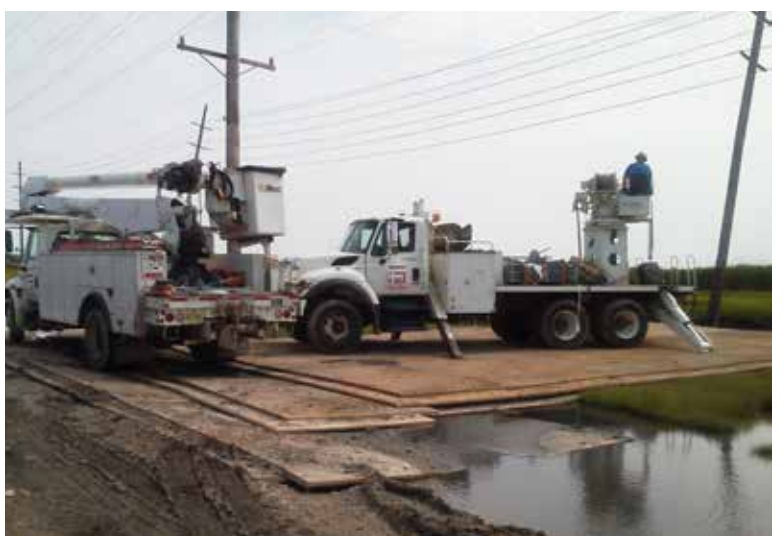
(Left and above): Work site access for pole replacement in New Jersey.
